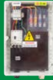
AC DISTRIBUTION BOX
